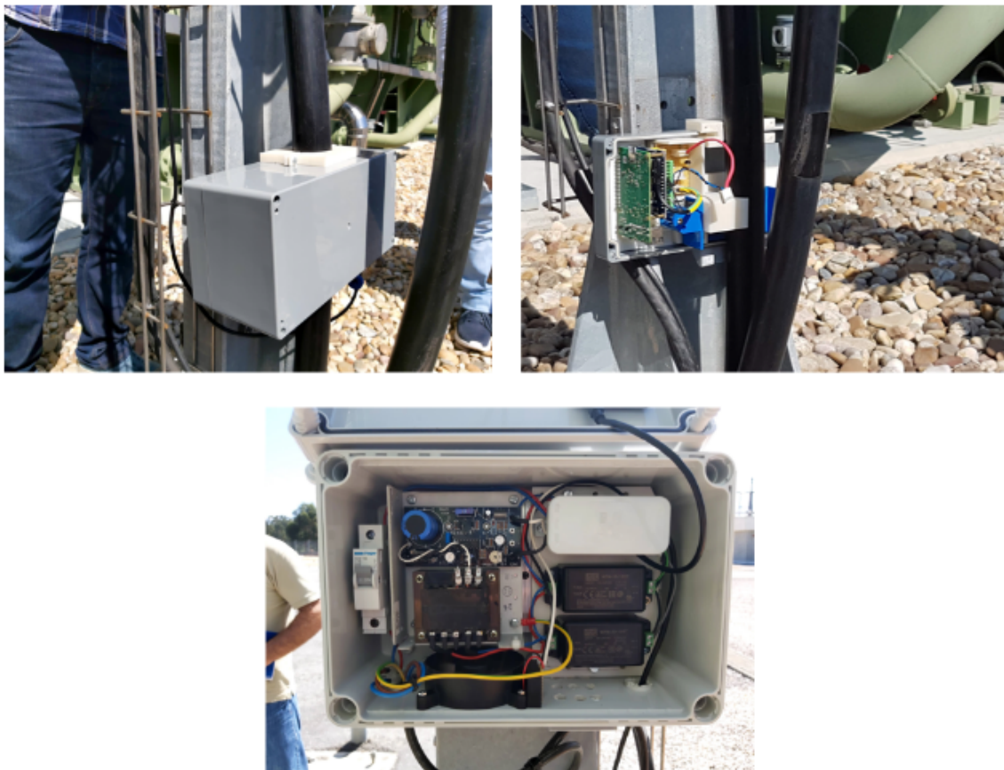
Figure 13. GIC instrumentation system for measuring GICs, installed at Paraimo substation. The system consists of two boxes: one with power sources (bottom photo), the other around the transformer neutral cable and the Hall effect sensor inside (two top photos).
